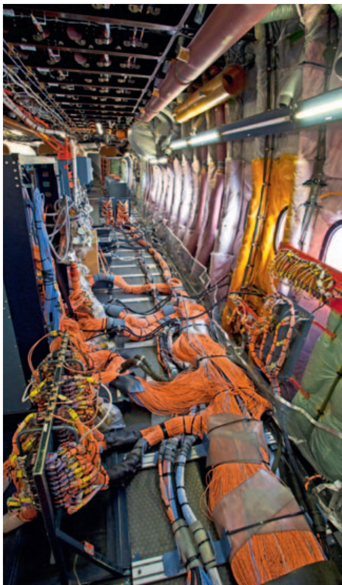
Unclad cabin in the Airbus A380 test plane: Cables and tubing lie exposed.
