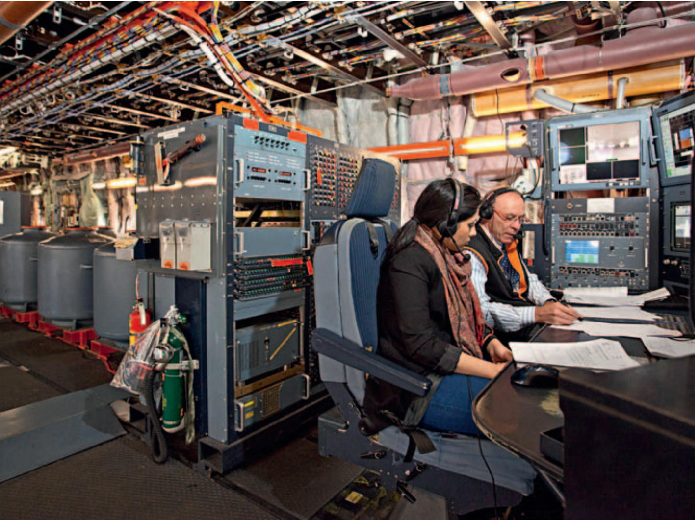
At the cabin's control station, test engineer Robert Ligné and his co-worker process data from 6,000 sensors and images from the outside cameras.
